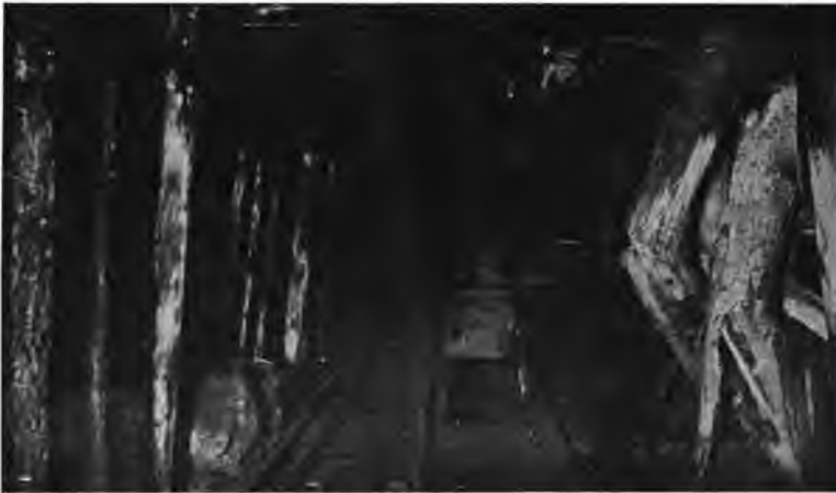
Fig. 13. Broken Timber in Gangway, G. Pabst Iron Mine, Ironwood, Mich.
